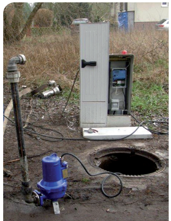
Installation of a sewage lifting system
